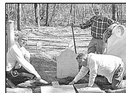
Members cement the SAR and DAR memorials a week before the service: Tony Beck, Frank Shorter and John L. Ramsey standing with a shovel.
